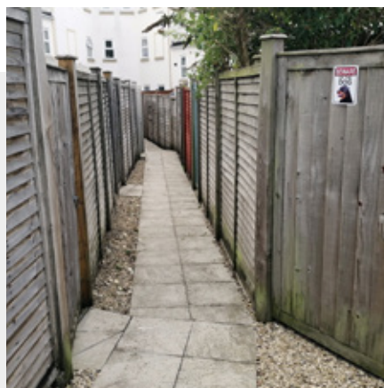
Insecure and unsafe access to housing area.
