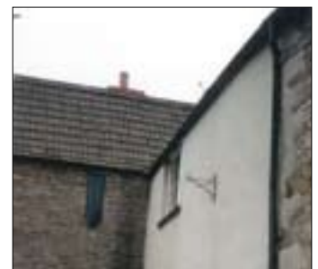
Stone quoins incorrectly expressed separately from the render. The render should be swept over the corners of the building, with no quoins.
