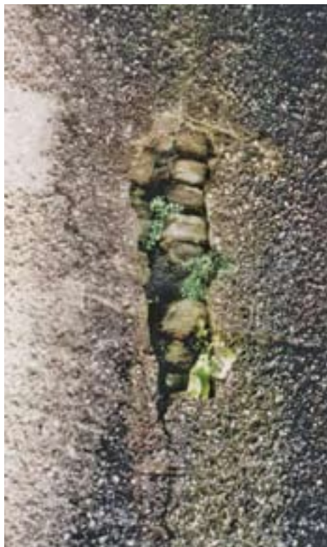
An example of cement render which has sheared away from the stonework, allowing water penetration and the growth of vegetation within the voids of the walling stone.
