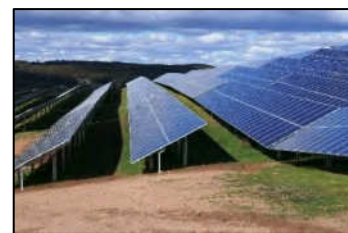
Figure 4: Ground Mounted Solar PV Array
