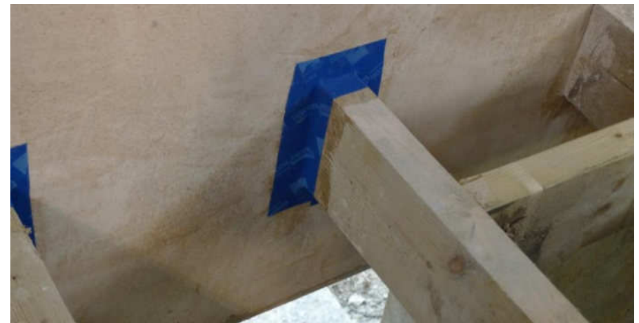
Applying airtightness tape to joist ends is a common measure required to achieve good airtightness in existing buildings. Large gaps may need filling with mortar first, and remember to apply a suitable primer.
