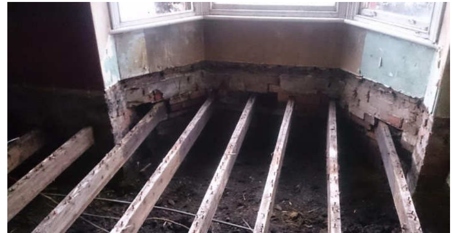
Achieving airtightness is possible in retrofit, but it is often necessary to strip back to the basic structure and perform basic repair work before methodically applying airtightness products and principles. Always consider risk of moisture and condensation.
