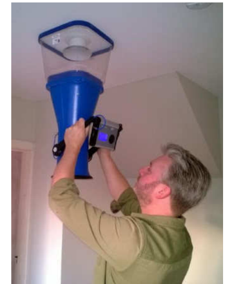
Flow rate measurement: image of MVHR system being commissioned (© Fourwalls)
