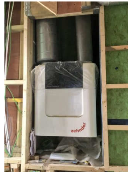
Image of Zehnder MVHR unit being retrofitted into an existing house (© Bowtie construction)
