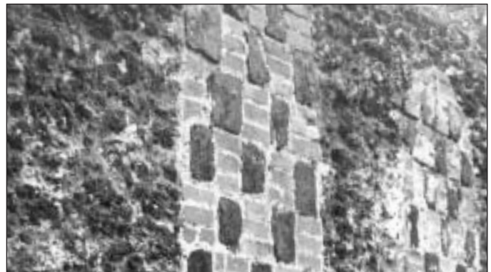
Detail of Chequered Wall - showing a mix of brick, slag and clinker.
