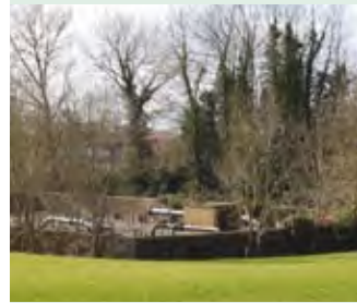
The unsightly gas installation would benefit from greater screening.
