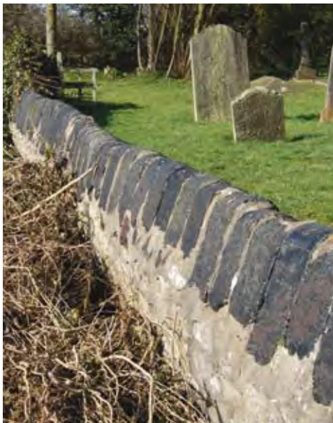
A stone boundary wall at St Anne's Church graveyard which features slag copings likely to have been sourced from the Warmley Brassworks
