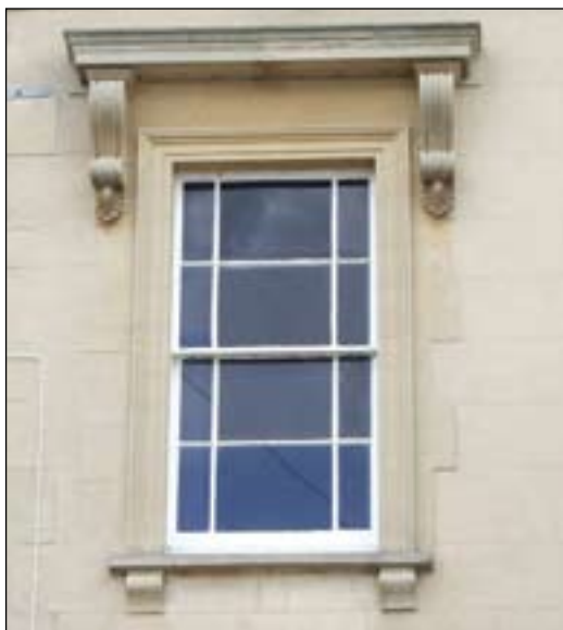
Sash window with marginal glazing and moulded stone surround on corbels, and hoodmould on decorative brackets.
