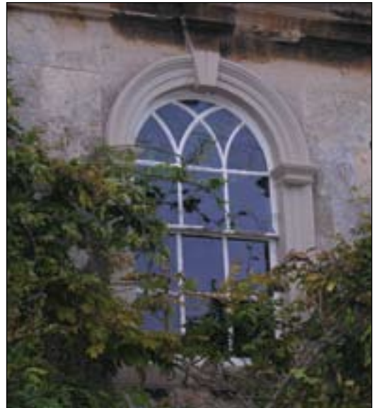
Early nineteenth century plain arched sash window with Gothic style glazing bar decoration.
