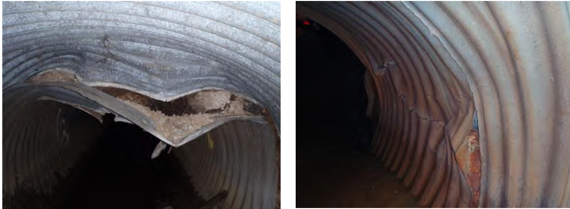
Photos of typical damage to Armco culvert (Note that these photographs were taken after the flood event and may not be reflective of the damage that was there at the time of the flooding)
