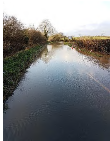
Figure 15 – Flooding at Perrinpit Road, Frampton Cotterell
