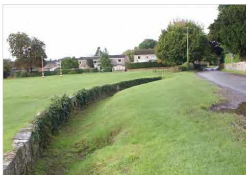
Parking and traffic has caused erosion of the verge.
