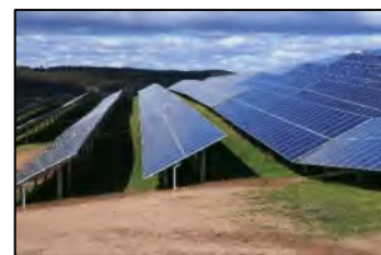
Figure 4: Ground Mounted Solar PV Array
