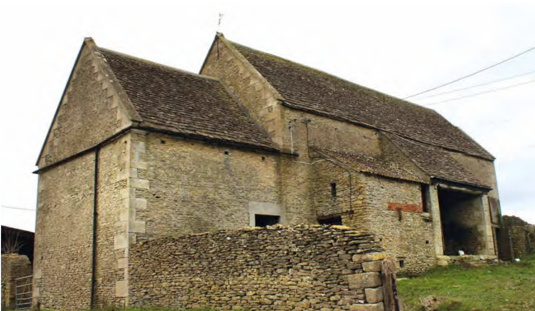
FIG.22 An existing barn pre-conversion. The open and informal character of its curtilage makes a positive and material contribution to its significance and should be preserved
