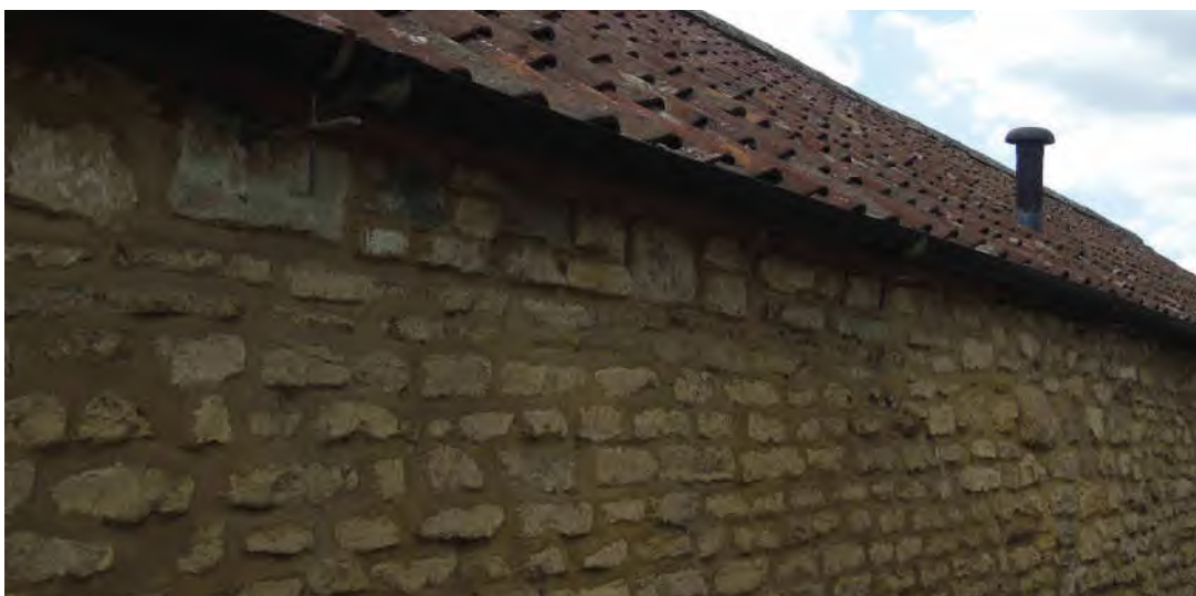
FIG.19 Traditional rise and fall brackets supporting the gutter
