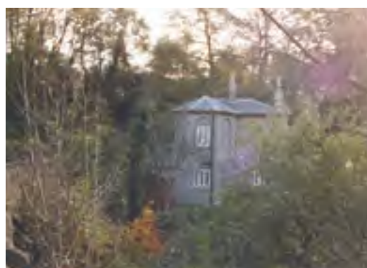
Overlooking the river the former lodge to Cleevewood House with its distinctive hipped slate roof. Care is needed over alterations.
