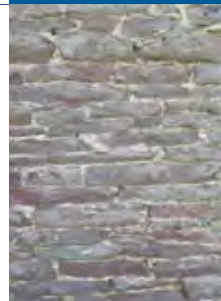
Wall pointed with lime mortar. The mortar is old but not failing and does not need to be replaced.
