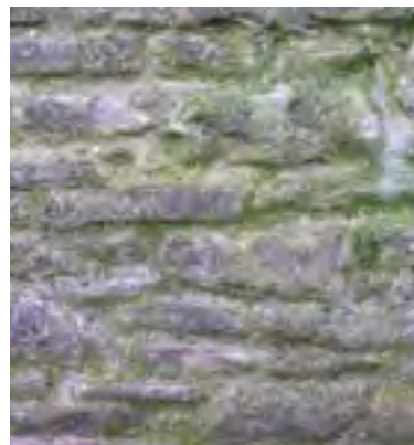
Manure has been applied to the new lime mortar pointing in order to encourage algae growth which will 'age' the appearance of the new pointing.
