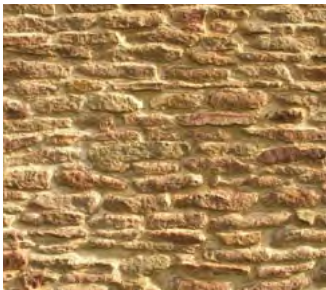
New lime mortar pointing correctly finished. The mortar is slightly recessed from the face of the stone, and brushed and tamped back to create an open texture and expose the aggregate.
