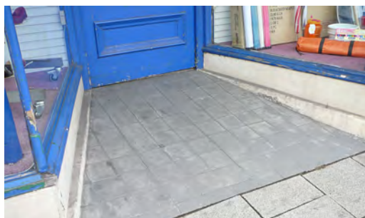
This entrance has been relaid to remove the step. Care should be taken with architectural features to avoid harming the shopfront design.
