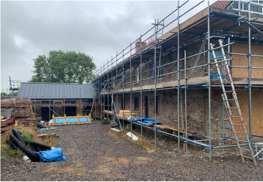
Figure 5: A self-build dwelling in progress located on a rural site, on the outskirts of Yate (Ref. PK18/4475/F). The form of the property has been inspired by local rural farm buildings with contemporary elements
