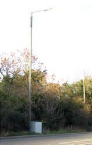
Electricity pylons and lamp poles can make suitable locations for antennas.
