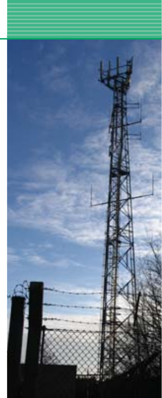
Poorly planned & sited telecoms masts can have a detrimental effect on views.
