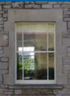
Traditional nineteenth century timber vertical sliding sash window with marginal glazing and slender glazing bars.
